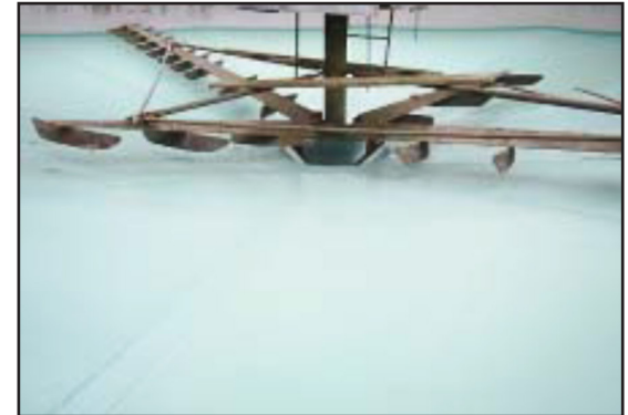
ARC S2 still in excellent condition
