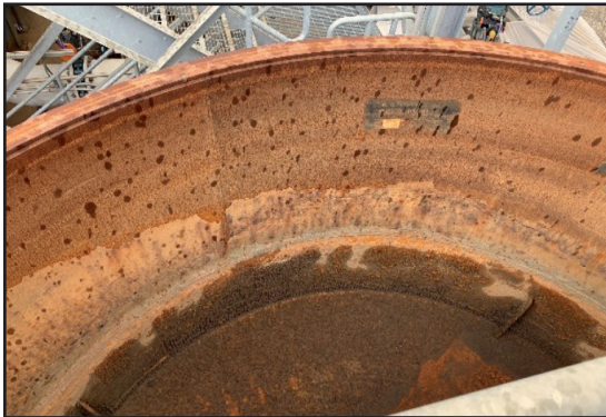
Severe corrosion inside tank [or] the bin.
